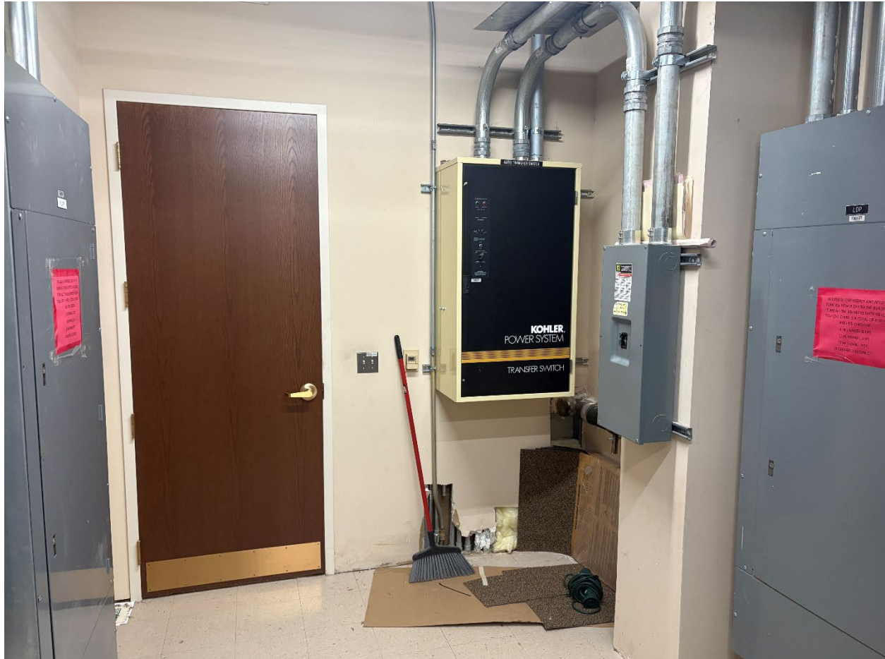
Photo #1 ATS Cabinet Location
