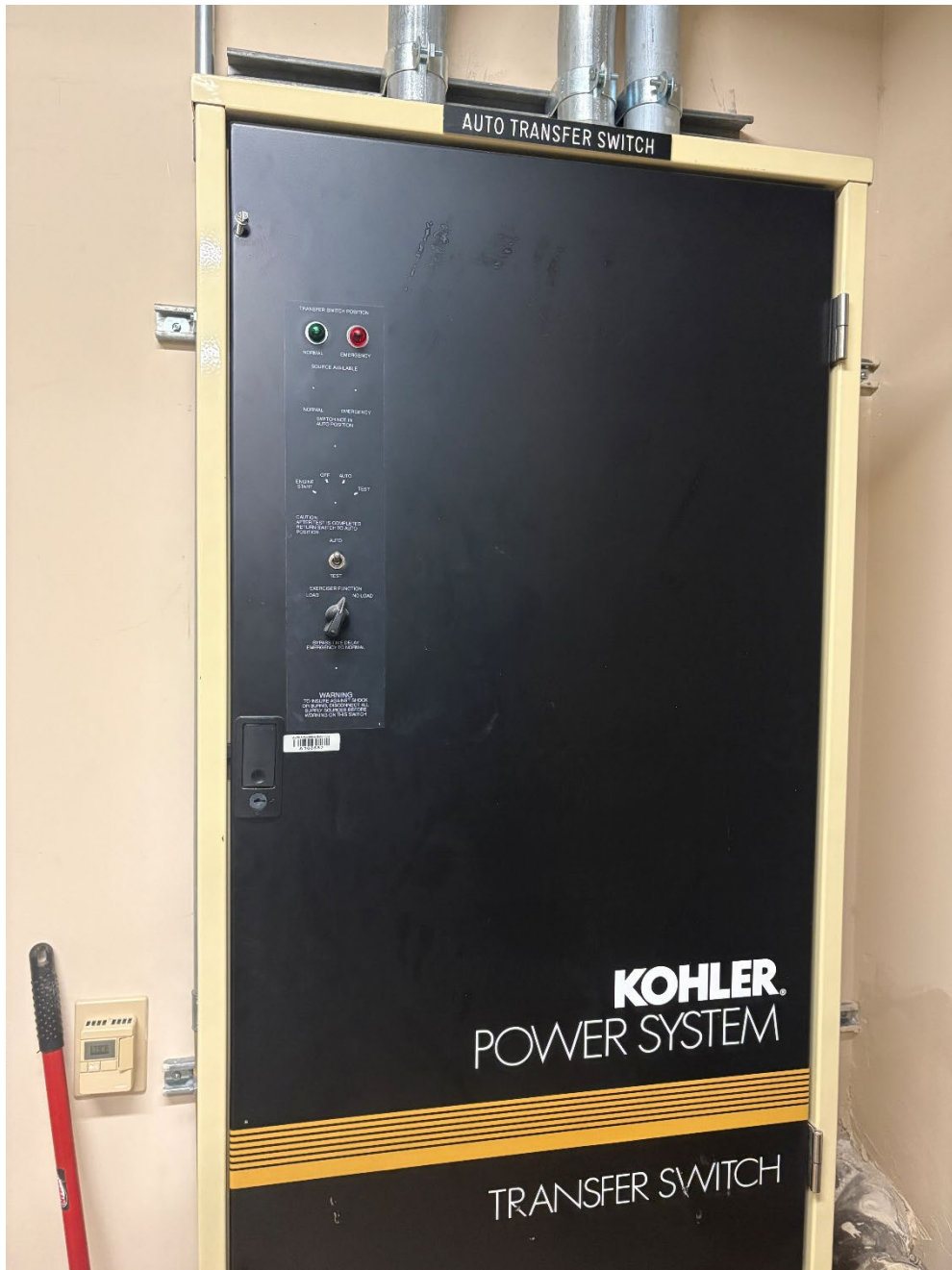
Photo #2 ATS Cabinet
