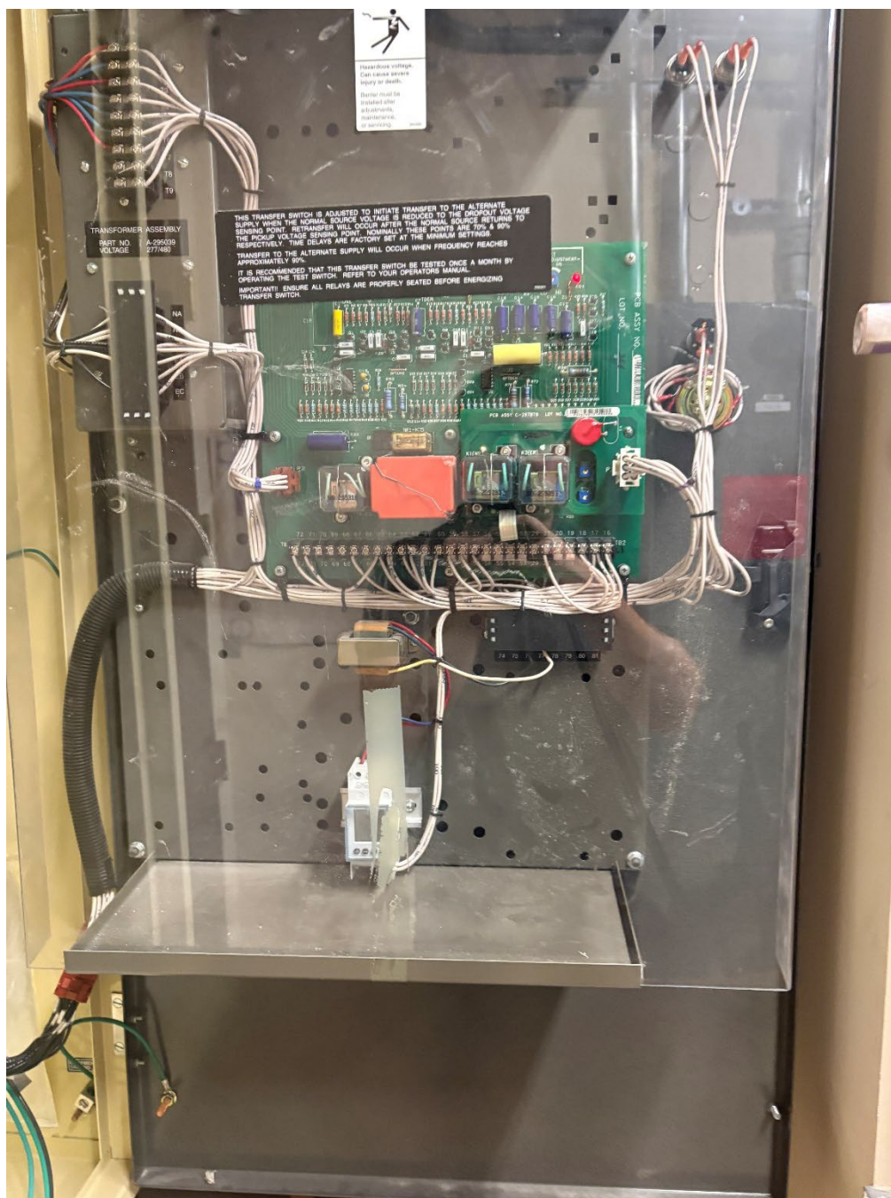
Photo #3 Back of Cabinet Door
