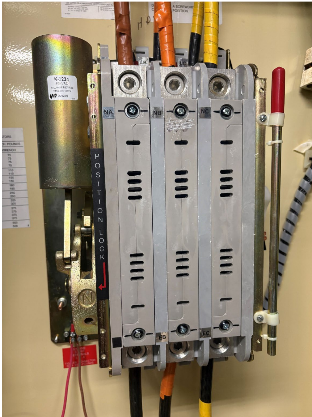
Photo #5 Cabinet Interior 2
